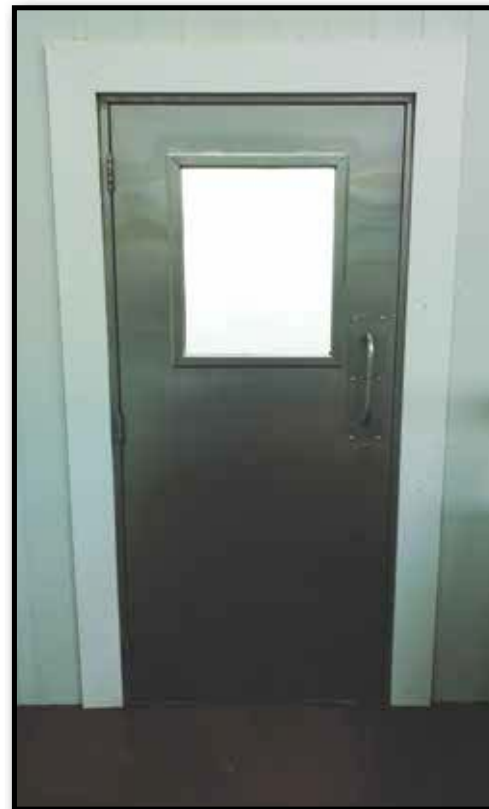
SS DOOR IN CHANNEL FRAME
